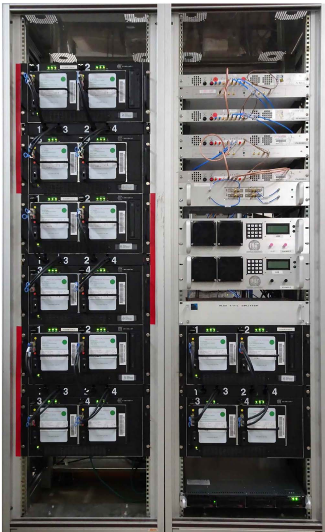
Figure 8. EHT digital VLBI backend as installed at the Institut de Radioastronomie Millimétrique (IRAM) PV 30 m telescope in Spain. The upper portion of the right-hand side rack holds the four R2DBE units. Two block downconverters are installed near the middle. The VLBI backend computer is mounted on the bottom right. The rack on the left and the lower portion of the rack on the right hold the four Mark 6 recorders with four disk modules each, providing a total of about 1 PB in data storage.
