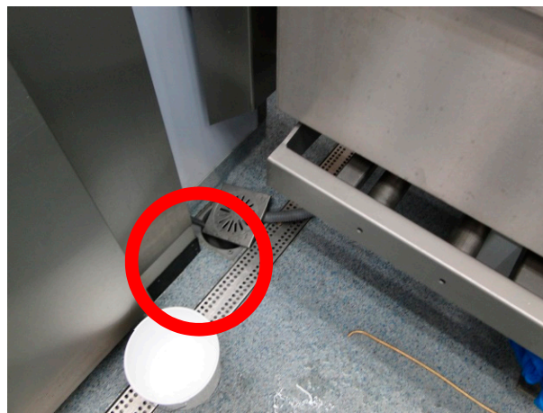
Figure 6. In the storage room the DFV system was blocked (red circle), preventing a free flow of air from the plenum to the extraction vent (T-4 in Table 2). Note that the grid in the floor is not for extraction of air; it is used to drain liquid spills.
