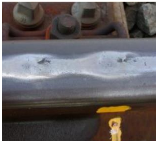
Figure 1.7: Squats formed on a normal grade rail track [62].
