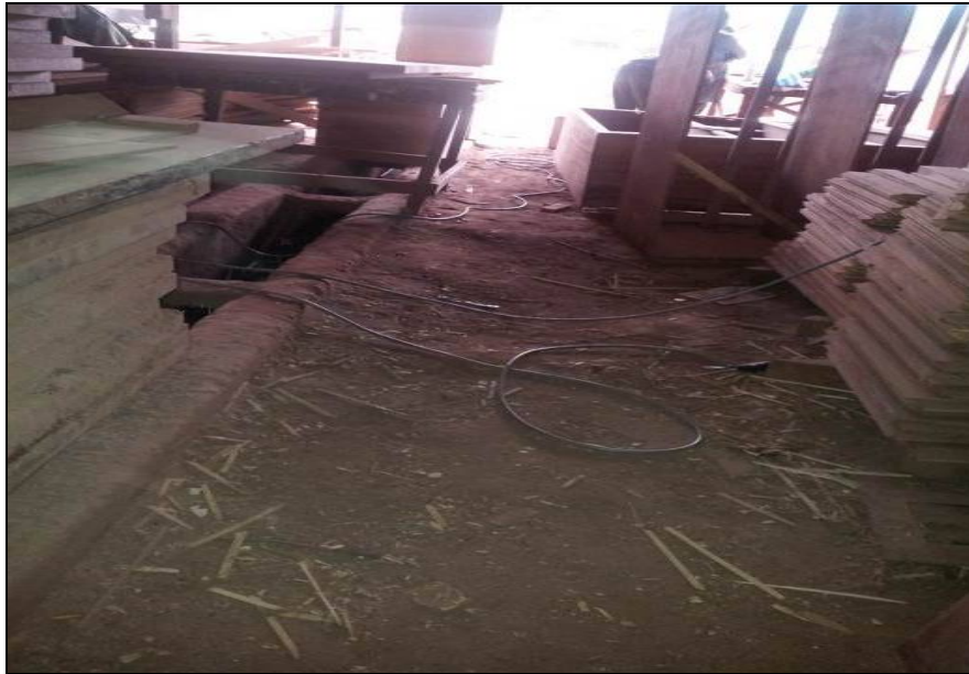
Figure 5.8 A photograph depicting electrical cables and packed wood obstructing the narrow walkways that can cause workers to stumble and fall resulting in serious injury
