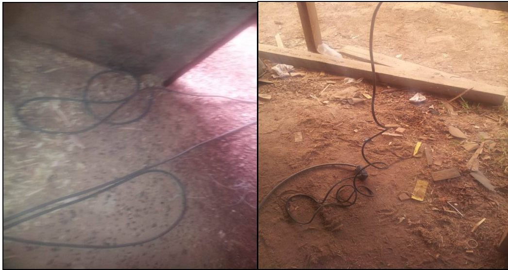
Figure 5.16 Photographs showing unsafe electrical connection and trailing electrical wires exposing workers to high risks of electrical shock
