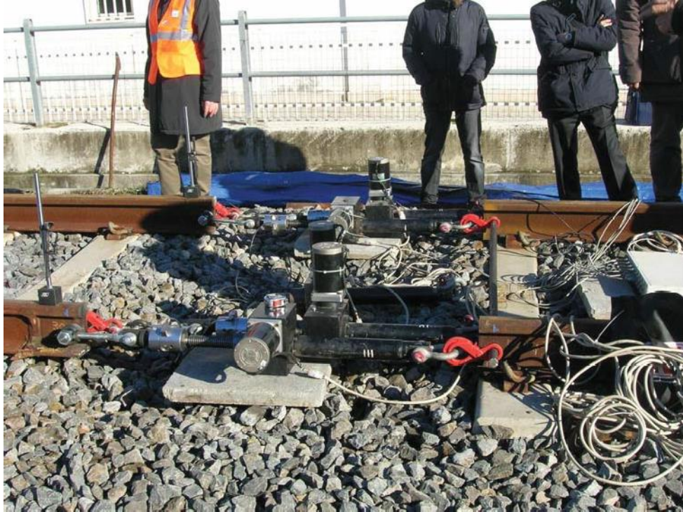
Figure 10. First longitudinal pull test: details of the actuators and their connections to the rails. FIGURE #10 219x164mm (300 x 300 DPI)
