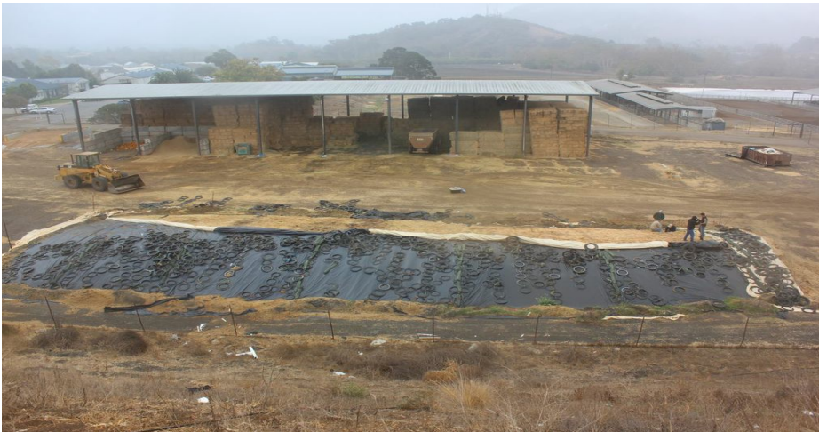
Figure 8. The OB film and Std plastic covers being removed from the pile.
