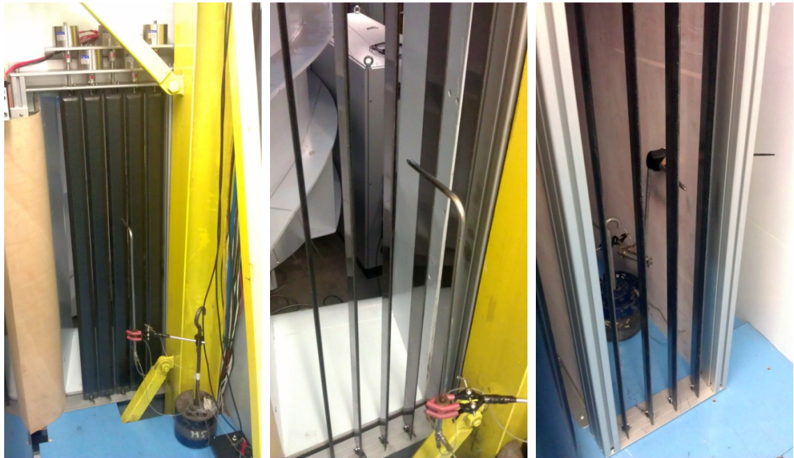
Figure 249 - Pitot-static tube mounting location on the downstream side of the front Y+ inlet duct
