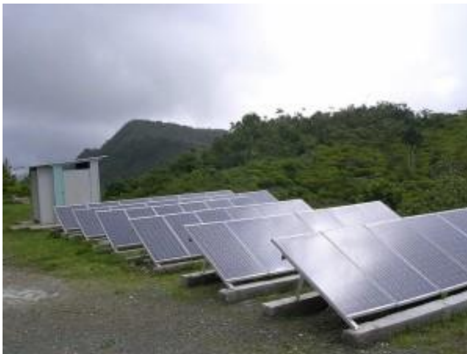
Picture 5. Solar panels in Cantarana (Photo by International Rivers).
