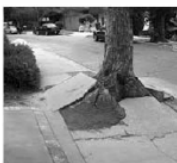
Less than 25% in Good Condition
