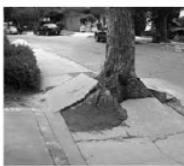
Less than 25% in Good Condition
