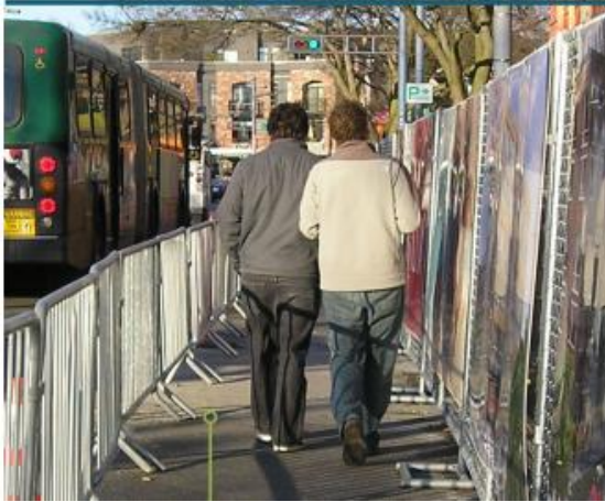
a) Pedestrian pathway separated from work zone and live traffic by using fences (Hawaii 2013)
