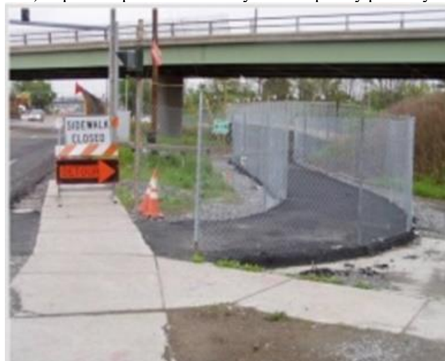
b) Temporary pathway is provided around the road in Greece town (Rochester, NY)
