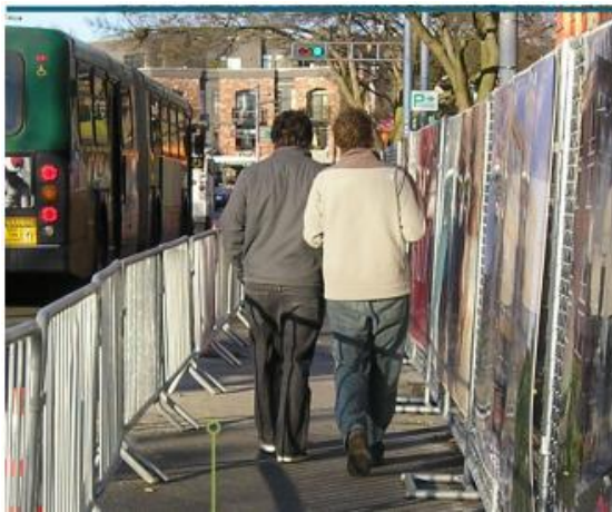
a) Pedestrian pathway separated from work zone and live traffic by using fences (Hawaii 2013)
