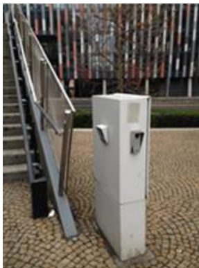
a) Pushbutton to call the platform
