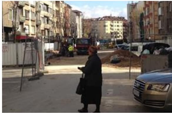
a) Complete street closure due to construction activities (non-motorized access parallel to the street is provided using the walkways located between the buildings and the work zone)
