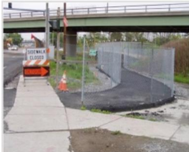
a) A temporary pathway is provided around the construction zone in Greece town (Rochester, NY)
