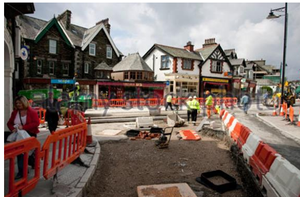
Figure 2-4. Railing as protective barriers (Google image)
