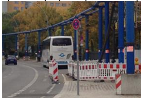
e) A temporary walkway with an uneven surface condition (Berlin , Germany)
