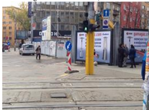
c) Unprotected non-motorized access provided in front of the work zone entrance
