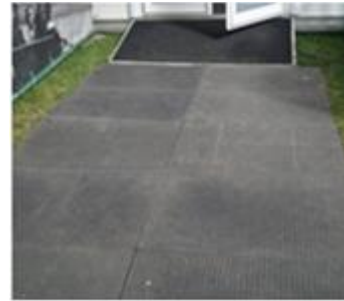
d) GT Trax (Groundtrax Systems Ltd 2017)
