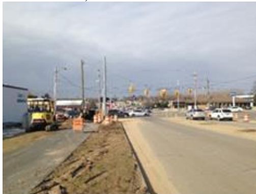
b) Closed sidewalk/trail connector on Romence Road Parkway (Picture 1)
