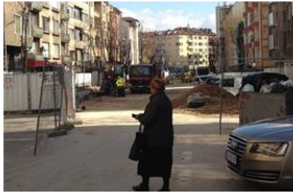
a) Complete street closure due to construction activities (non-motorized access parallel to the street is provided using the walkways located between the buildings and the work zone)
