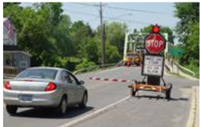
b) Automatic Flagger Assistance Devices (AFAD) is used to control motorized traffic
