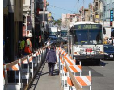
b) A travel lane used to provide access to pedestrians due to work on the sidewalk (Google image).
