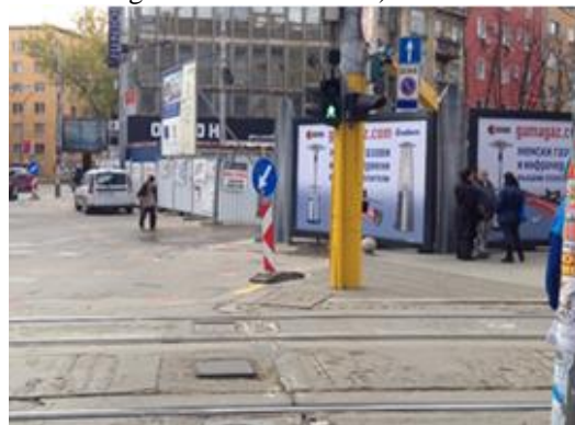
c) Unprotected non-motorized access provided in front of the work zone entrance
