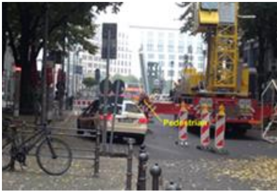
b) A pedestrian standing next to the crane and waiting to pass through the construction zone
