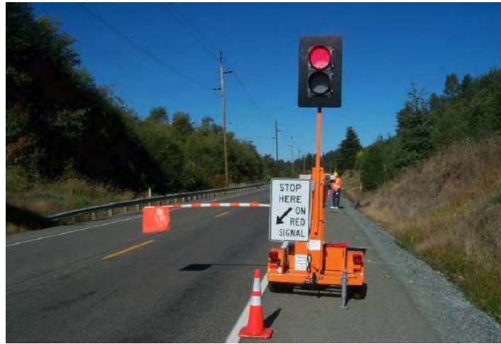
b) Temporary traffic control devices
