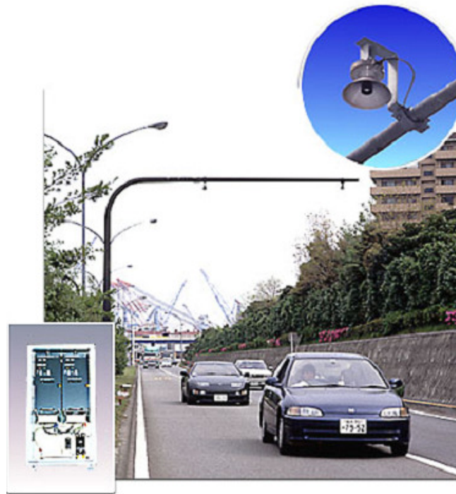
Figure 3.3: Ultrasonic sensor-based traffic monitoring system mounted on an overhead structure [13]
