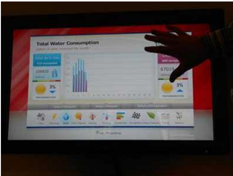
Figure 11: 32-inch Touch Screen Water & Electricity Monitor in Likins Hall
