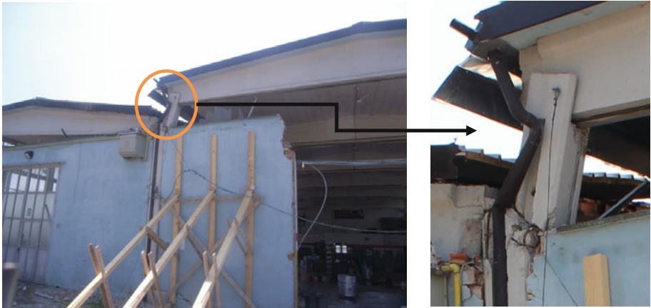
Fig. 10 Loss of the left girder seating due to the interaction with masonry panels (short columns/shear failure)
