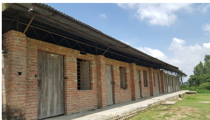
Fig. 4. Picture of a masonry school building in Nepal, Copyright: Kapil Khatri, Submitted to the SAFER Project Mobile App.
