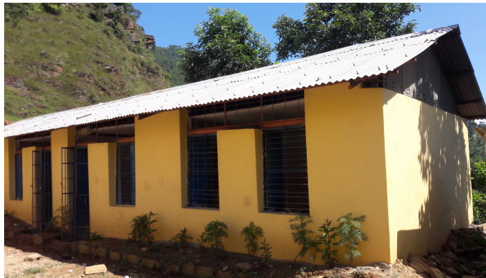
Fig. 3. Picture of a steel school building in Nepal, Copyright: Amar Khamcha, Submitted to the SAFER Project Mobile App.
