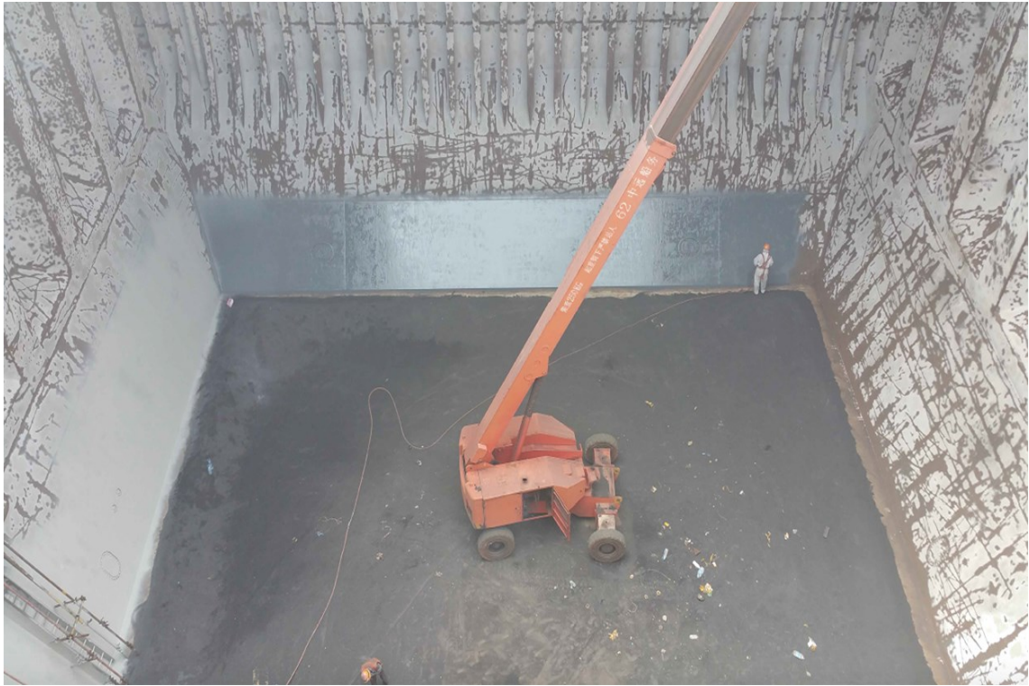
Figure 40 - Application of EZR Primer on board No.4 (P) Cargo Hold of Post Panamax Bulker – Case A
