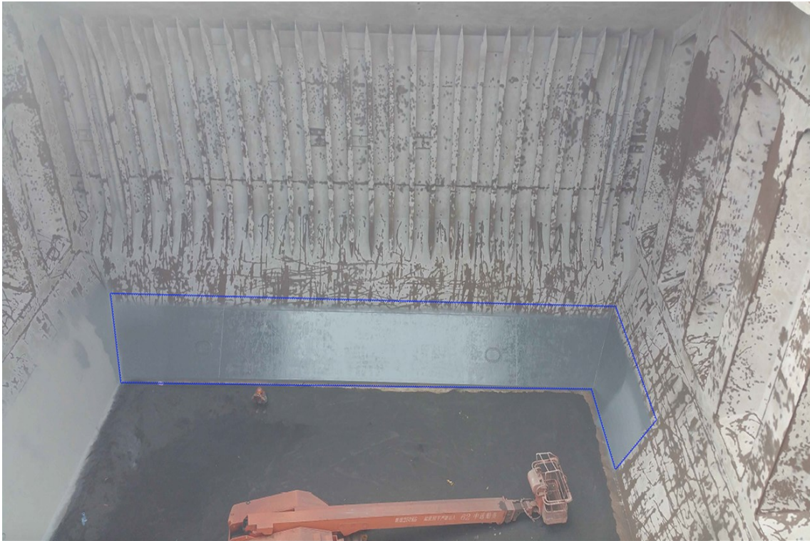
Figure 42 - Completed application of EZR Primer on board No.4 (P) Cargo Hold of Post Panamax Bulker – Case A . Blue line denotes application area.
