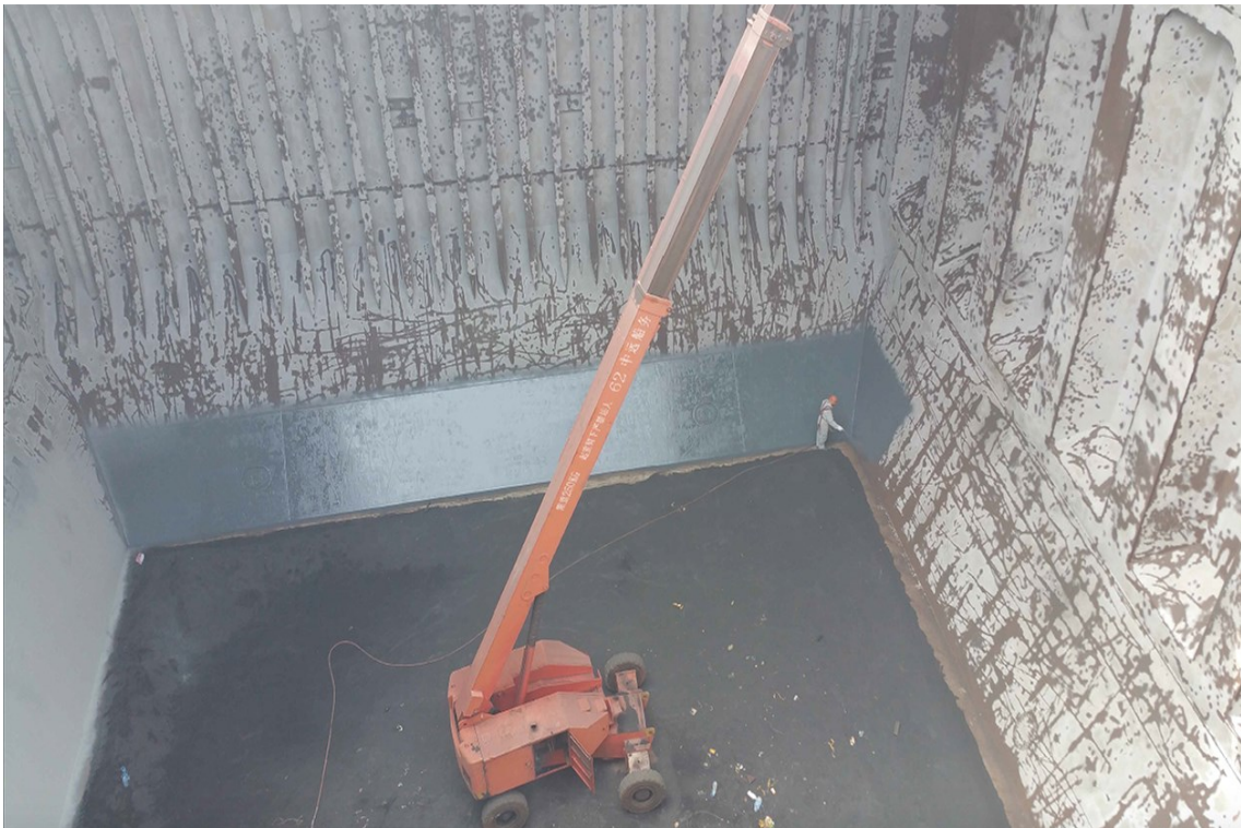
Figure 41 - Application of EZR Primer on board No.4 (P) Cargo Hold of Post Panamax Bulker – Case A
