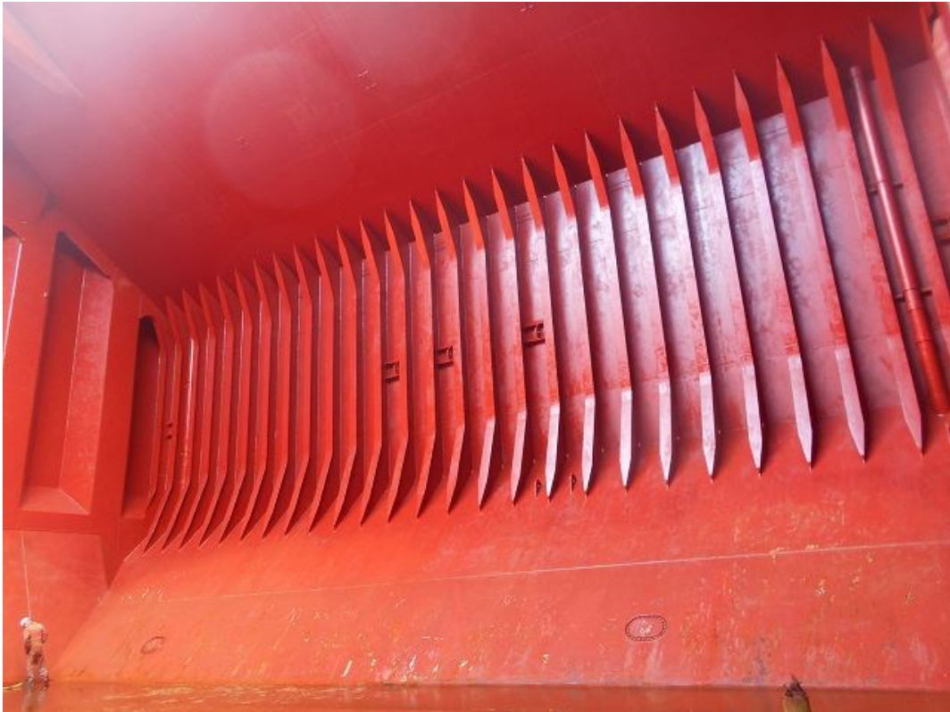
Figure 47 - Port Side of No.4 Cargo Hold of Post Panamax Bulker, 16 months after application of Epoxy N coating.
