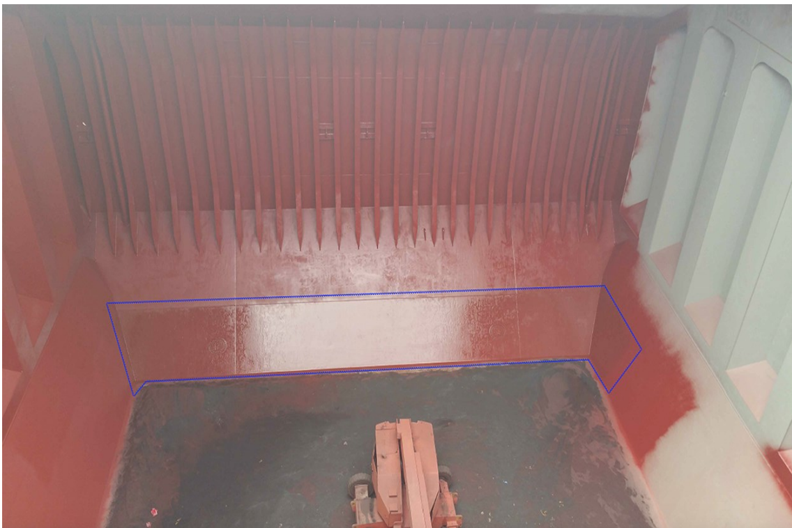
Figure 43 - Application of Epoxy N top coating on board No.4 (P) Cargo Hold of Post Panamax Bulker – Case A. Epoxy N appears glossier than surrounding coatings. Blue line denotes application area.
