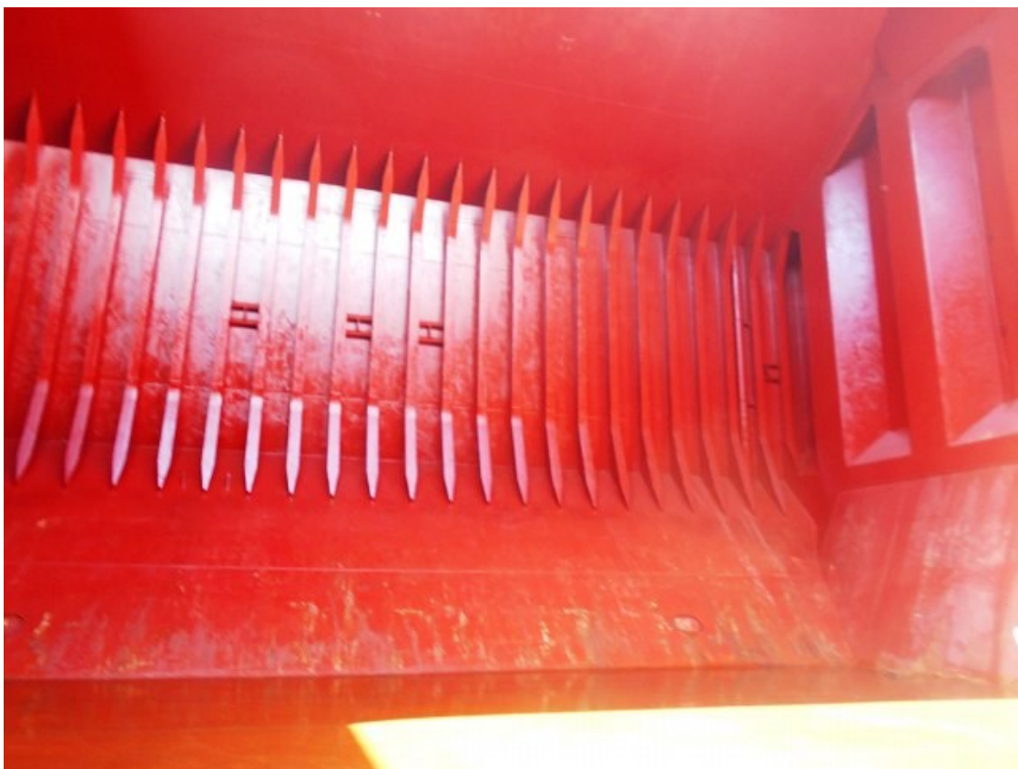
Figure 48 - Starboard Side of No.4 Cargo Hold of Post Panamax Bulker 16 months after application of Epoxy B coating.
