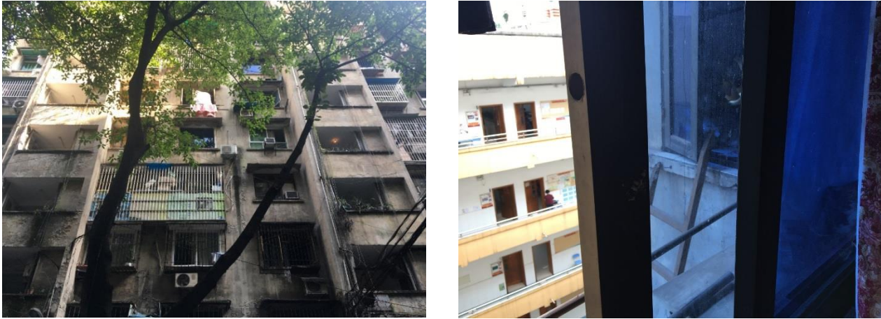
11 Figure 7. Outside view of the building (on the left) and detail of the sliding window (on the right)
