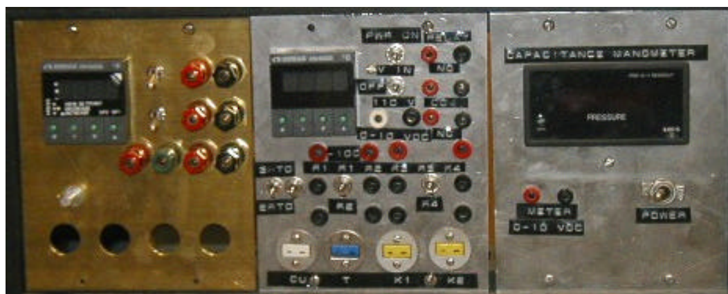
Fig. 2.11. Left and center portions of the photograph showing the temperature controls units.
