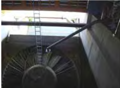
View of the injection tube connected to a strut installed on the VLH wicket gate. © Ecogea
