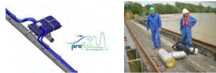
ProFish repulsion system installed on floats in the flume supplying the Biron hydroelectric plant. (Image © ProFish, photo © F. Travade)
