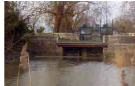
The Charras installation (tide gates closed for high tide) seen from downstream. © P. Baran
