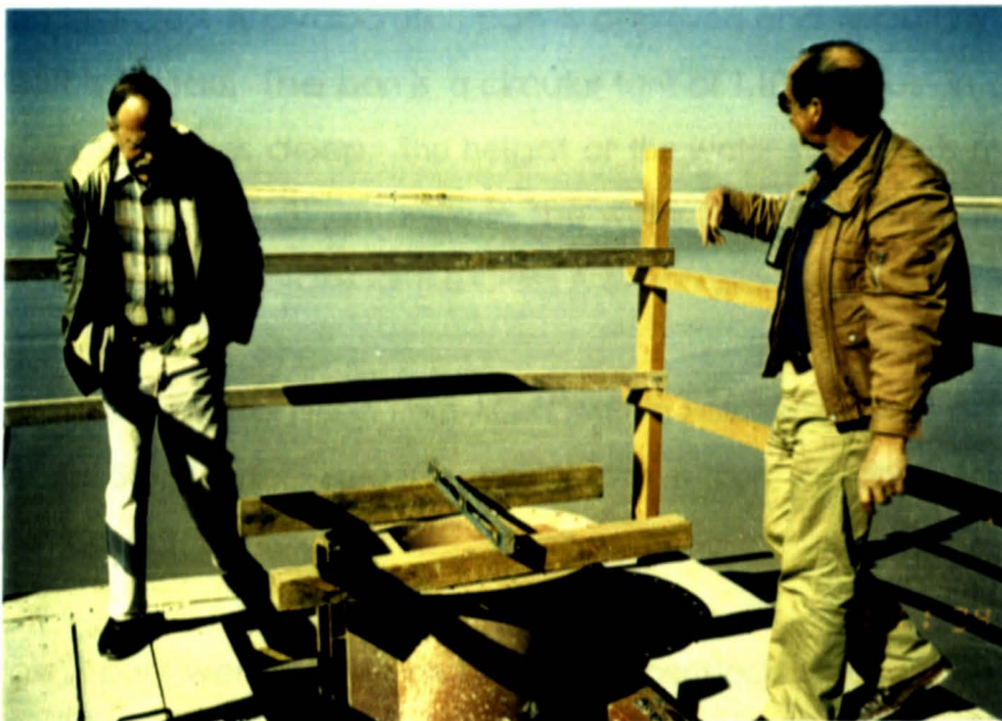
Figure 11 : Preparing the penstock pipe for a level base for the Class A pan.
