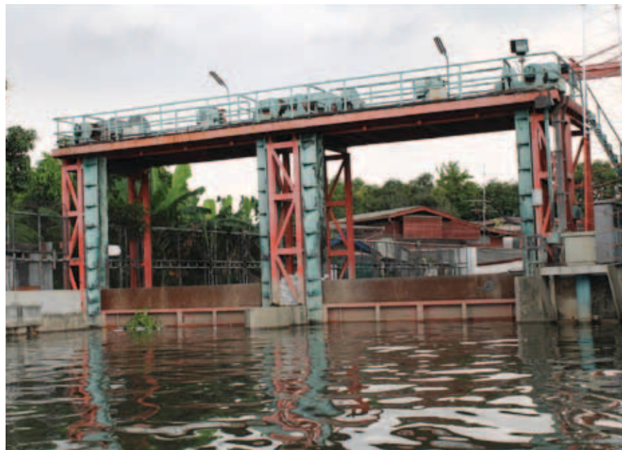
Flood water almost reaching the maximum level. Bangkok, Thailand
