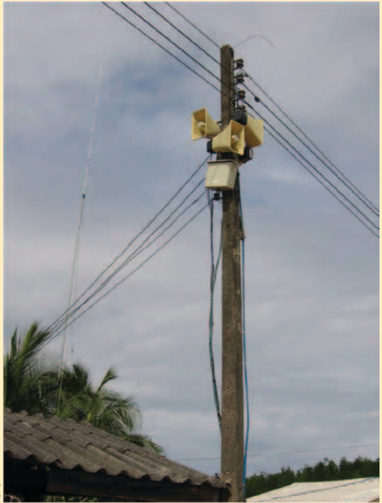
Loudspeakers installed as part of actions to strengthen community early warning systems. Thailand
