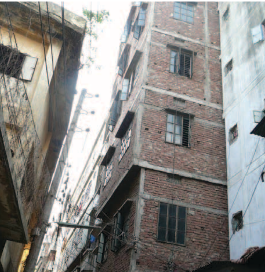
Vulnerable buildings contribute to increased disaster risk in urban areas. Dhaka, Bangladesh
