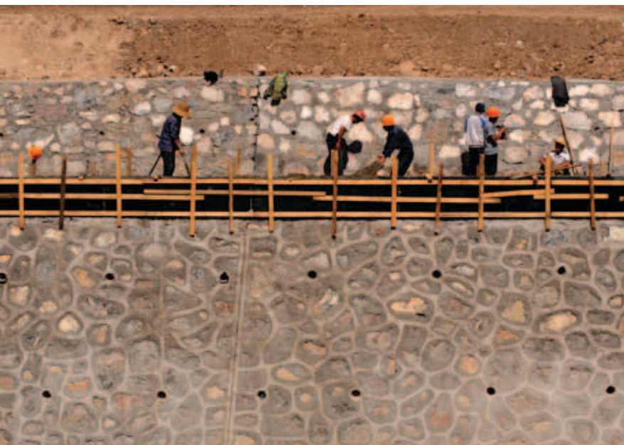
Diversion channels being constructed to reduce risk from floods and mudslides. Gansu Province, People's Republic of China
