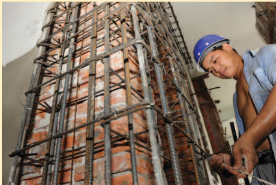
A construction worker reinforces a school building. Hefei, People's Republic of China
