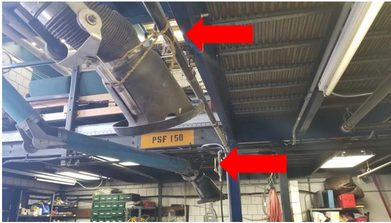
Figure B3. The hoods for the local exhaust ventilation system in the pipe fitter shop had been tied to pipes over workstations using ropes. Photo by NIOSH.
