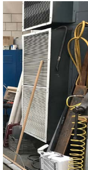
Figure B2. The air intake located in the northwest corner of the boat bay. Photo by NIOSH.
