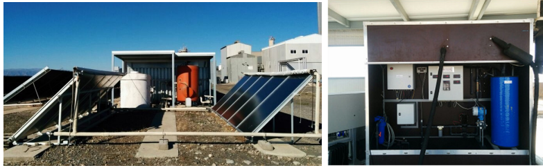
(a) SMD facility. (b) Solar Spring pilot module.
