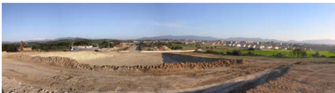
Fig. 4B.2 Panoramic photograph, facing north, of the site during the construction works of the railway infrastructure (photo by Rafel Rosillo, Arqueolític).
