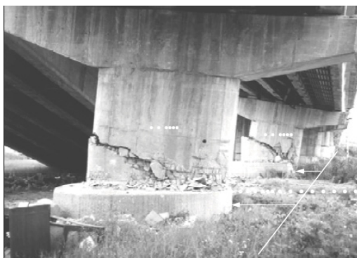
e) Shear failure of the piers of a bridge, Taiwan earthquake 1999
