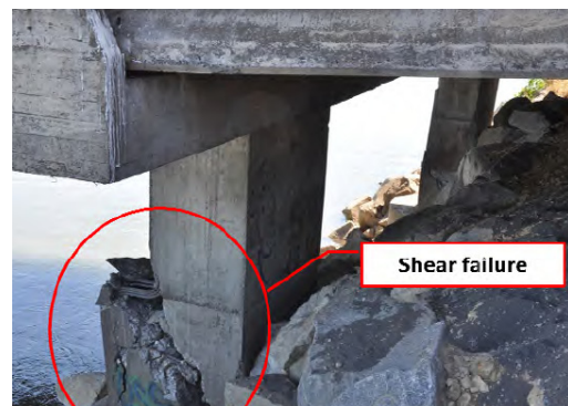
f) Pier shear failure of the bridge crossing Bio Bio River in Chile earthquake in 2010
