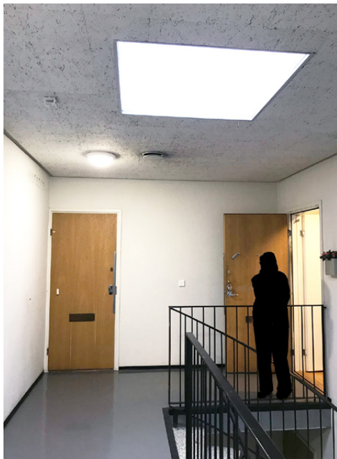
Image 10.7.3 A skylight above the staircase of a 1960s apartment building provides daylight into the stairwell.
