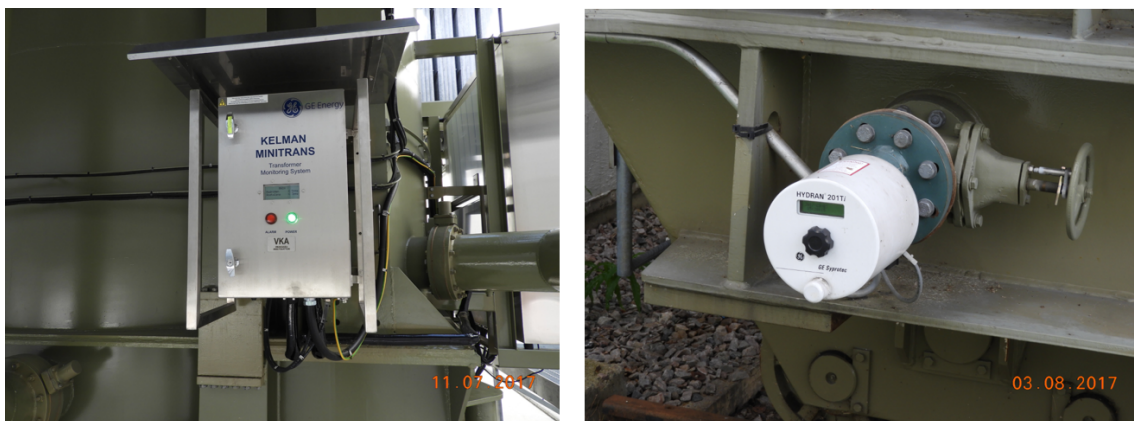
Figure 21: Equipment for continuous online DGA. [10]
