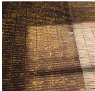
Figure 41 Steel grating, attacked by corrosion
