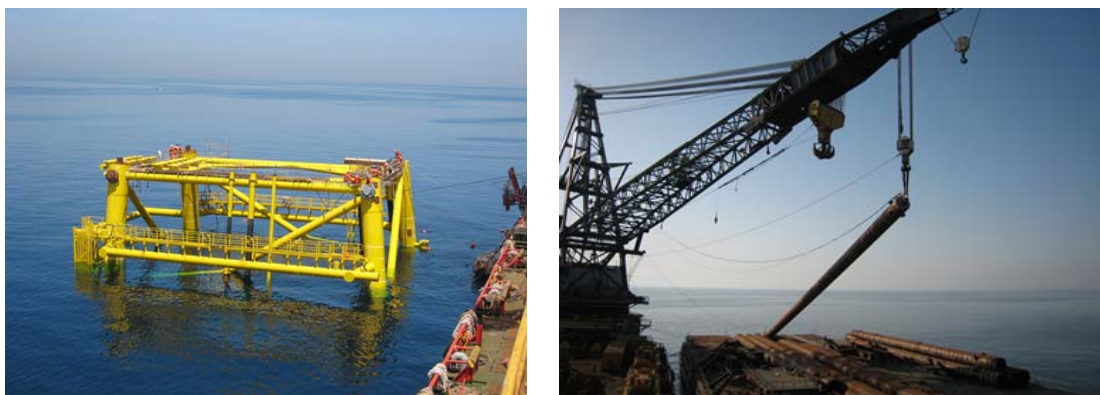
Figure 10 Picking up the pile from the barge's deck (Alyafei and Maerskoil Qatar, 2009)
