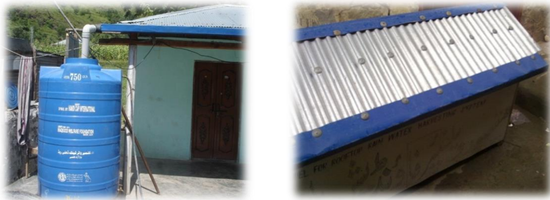
Figure 3. 9 Rooftop rainwater harvesting system in AJK Pakistan installed by ERRA
