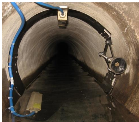
Figure 2: Temporary flow monitoring location OCM Pro (NIVUS) upstream WWTP
