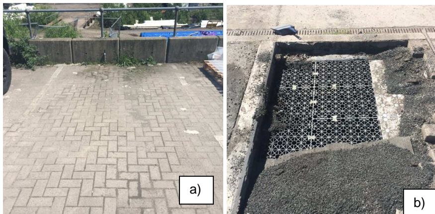
Figure 2. a) Interlocking porous paving car park bay excavated for this study from Bury. b) Excavation of the car park bay exposing the profile of a porous paving system.
