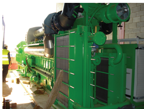
Figure 7.5 Heat exchangers for the recovery of thermal energy at the high temperature circuit
