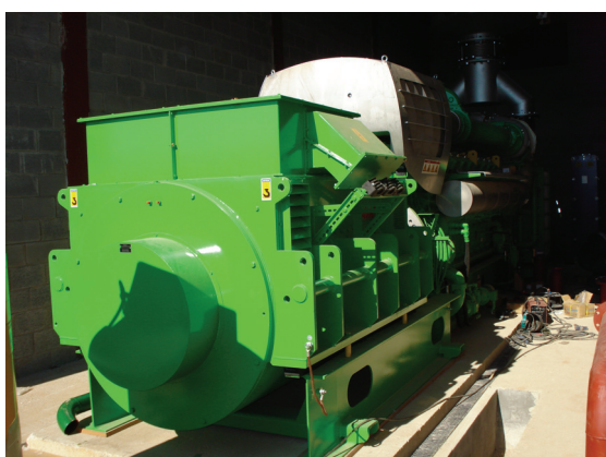
Figure 7.4 One of the Jenbacher engines, with its electric generator at the front of the picture
