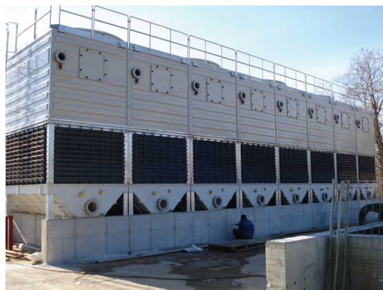
Figure 7.9 General view of the cooling towers
