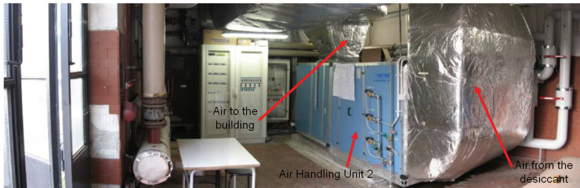
Figure 6.9 Control system and main air handling unit (AHU2) placed inside the utilities building
