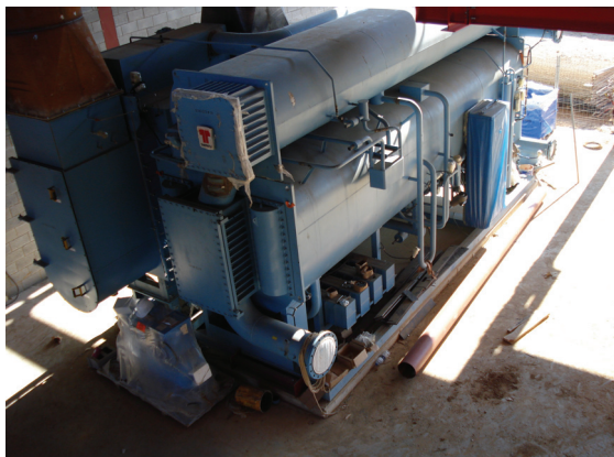
Figure 7.6 DE absorption chiller activated with exhausts gases coming from the cogenerators
