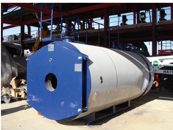
Figure 7.10 View of the backup boiler of 5 MW
