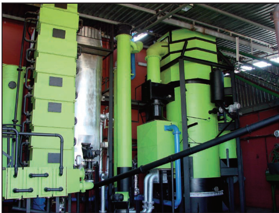
Figure 7.14 ENAMORA gasification plant (Gasifier+synthesis gas treatment)
