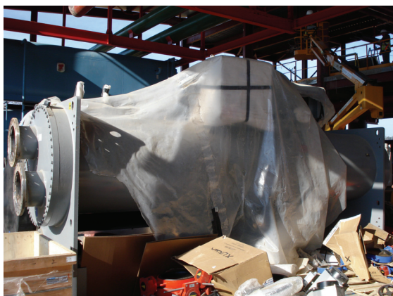
Figure 7.8 Electric chiller before being installed
