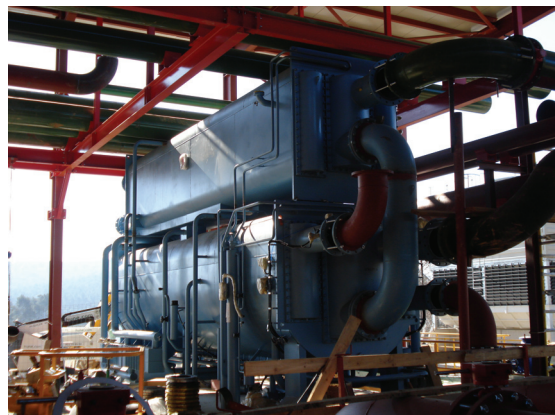
Figure 7.7 SE absorption chiller activated with the hot water produced with the cogenerators
