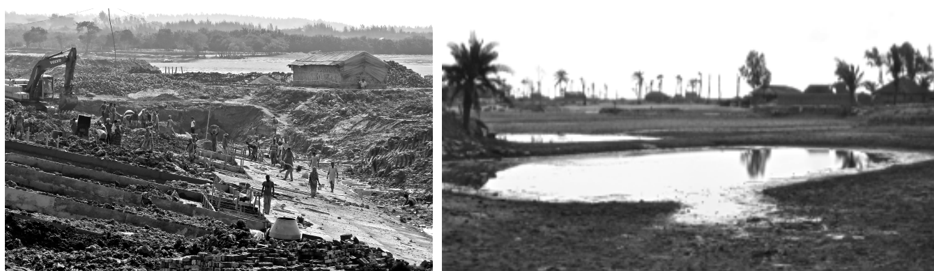
Figure 3 Large-scale embankment construction in Beguakhali (left). Remaining households in Dhablat unprotected by embankment (right)
