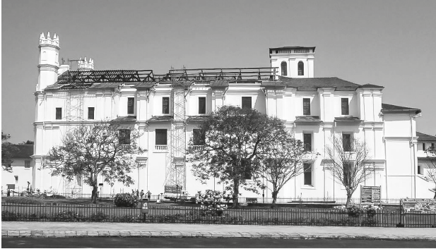
Image 1 – Church of Saint Francis of Assisi, in Old Goa, during an intervention by the ASI (source: Joaquim Rodrigues dos Santos)
