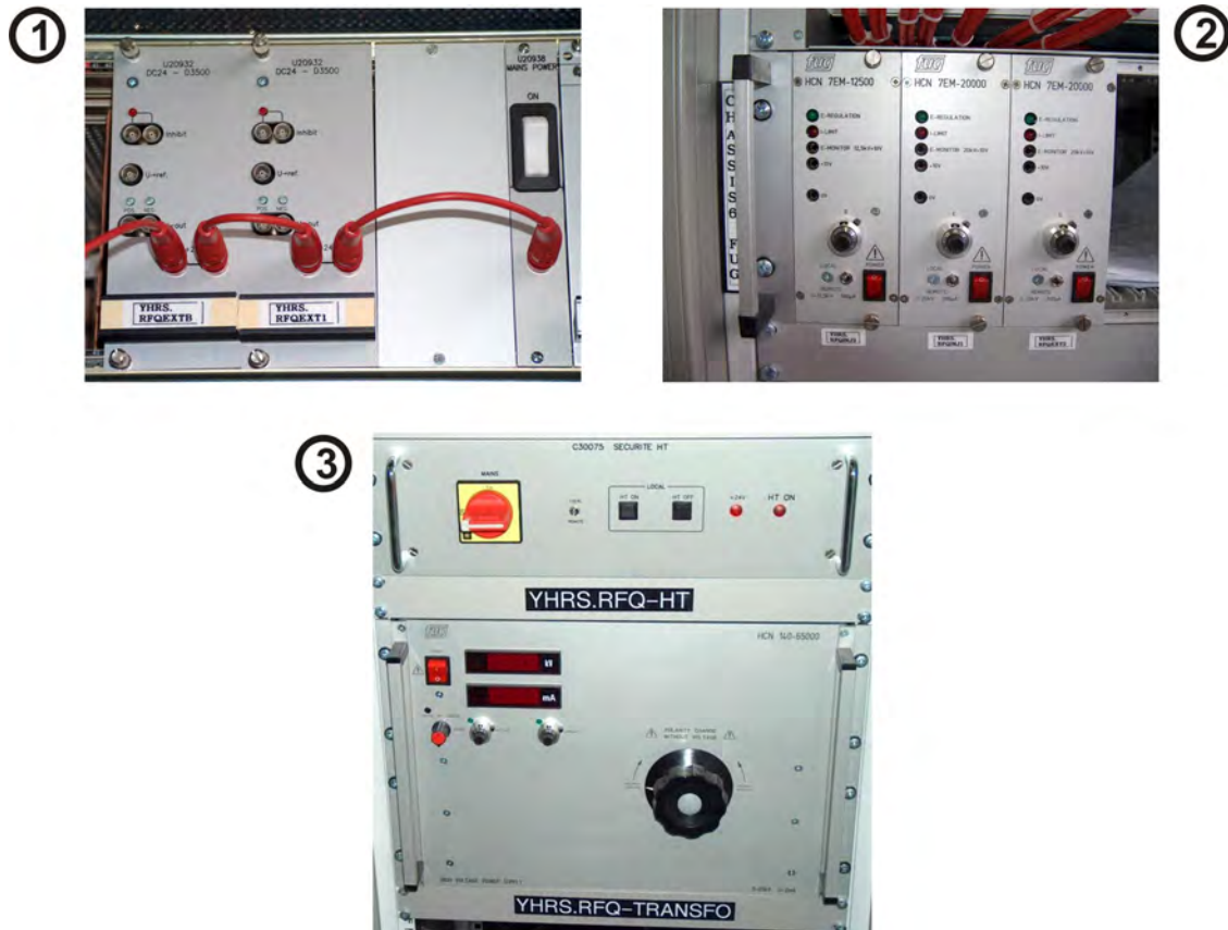
Figure 9.8: Pictures of the different DC power supplies for the ISCOOL system: 1) 0.5 kV DC power supplies, 2) 12.5 kV and 20 kV power supplies and 3) HV power supply up to 65 kV.
