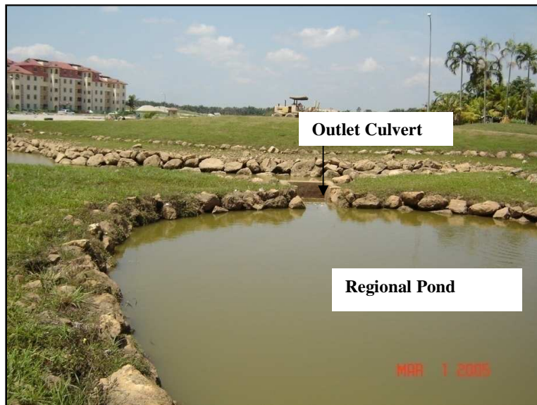
Figure 2.8: Regional Detention Pond in Kota Warisan, Bandar Baru Salak Tinggi, Selangor
