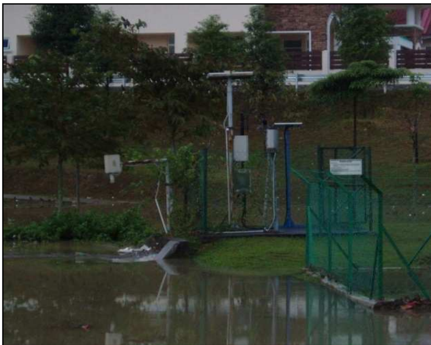
Figure 1.9: Condition at Pond Outlet/Culvert Inlet after Storm Event
