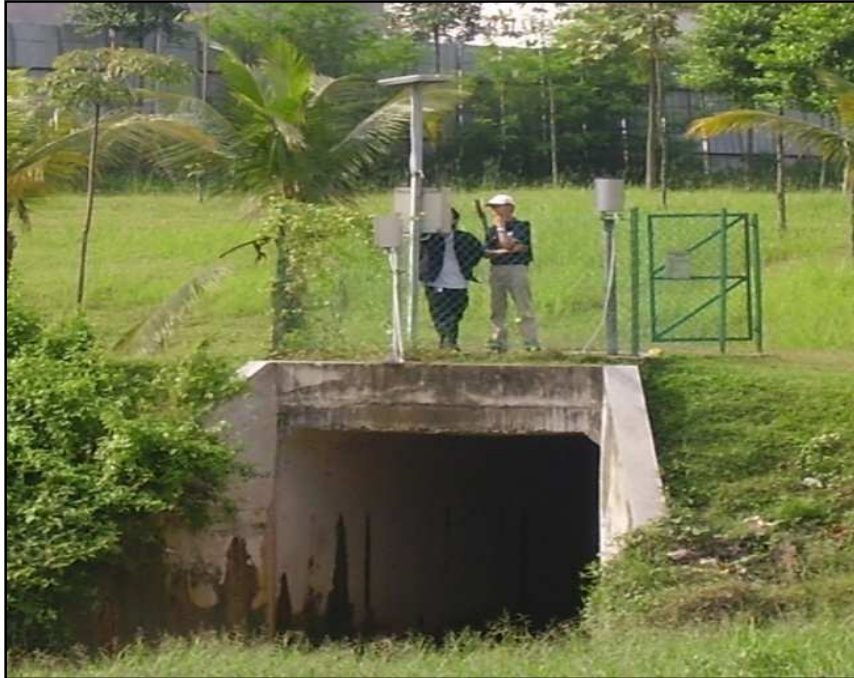
Figure 1.8: Condition at Pond Outlet/Culvert Inlet during Dry Season
