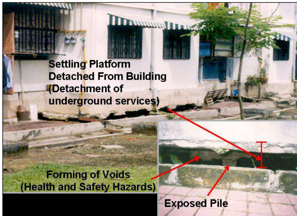
Figure 1.1 Problems for buildings with piled to 'set' foundation on soft ground
