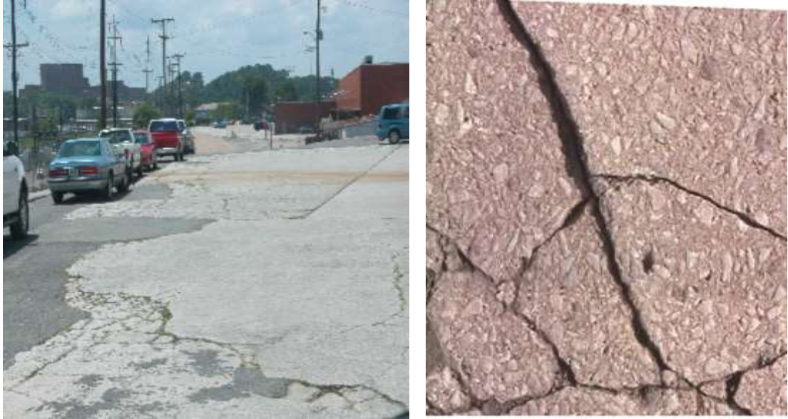
Figure 1.1. Image showing road cracking (Yu et al, 2005).
