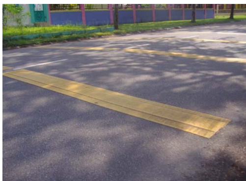
Figure 1.1 Typical TRS in Malaysia
