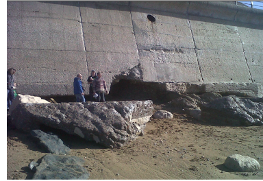
(b) Structural damage suffered at its toe during an event on the 5th February 2014 is clearly visible.
