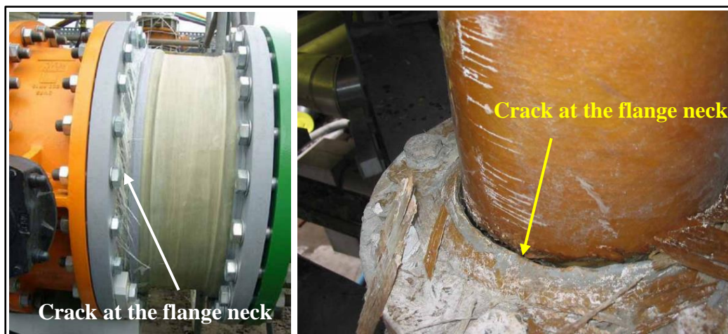
Fig. 4.5: Common failure on the GFRP flanges [33]
