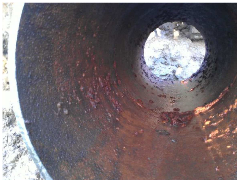
Fig. 1 The interior of a ductile iron main that was drained down to repair a leak. Note the thin (particulate) material coating the complete pipe wall, as well as larger more stable corrosion tubercles
