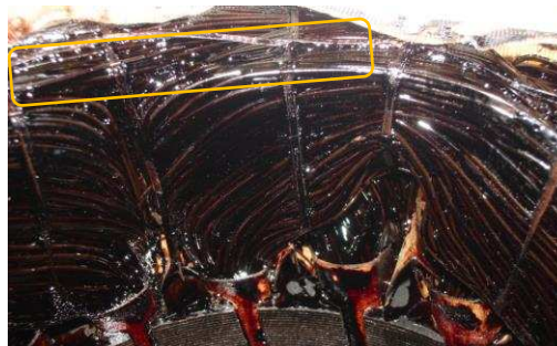
Fig. 10 Sample 3 End-Windings After Failure. Phase-phase overlap in the EW region is highlighted
