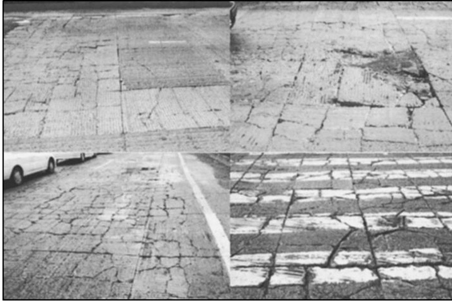
Figure 1.1. Failure of UTW in Taiwan (After Lin & Wang [3])
