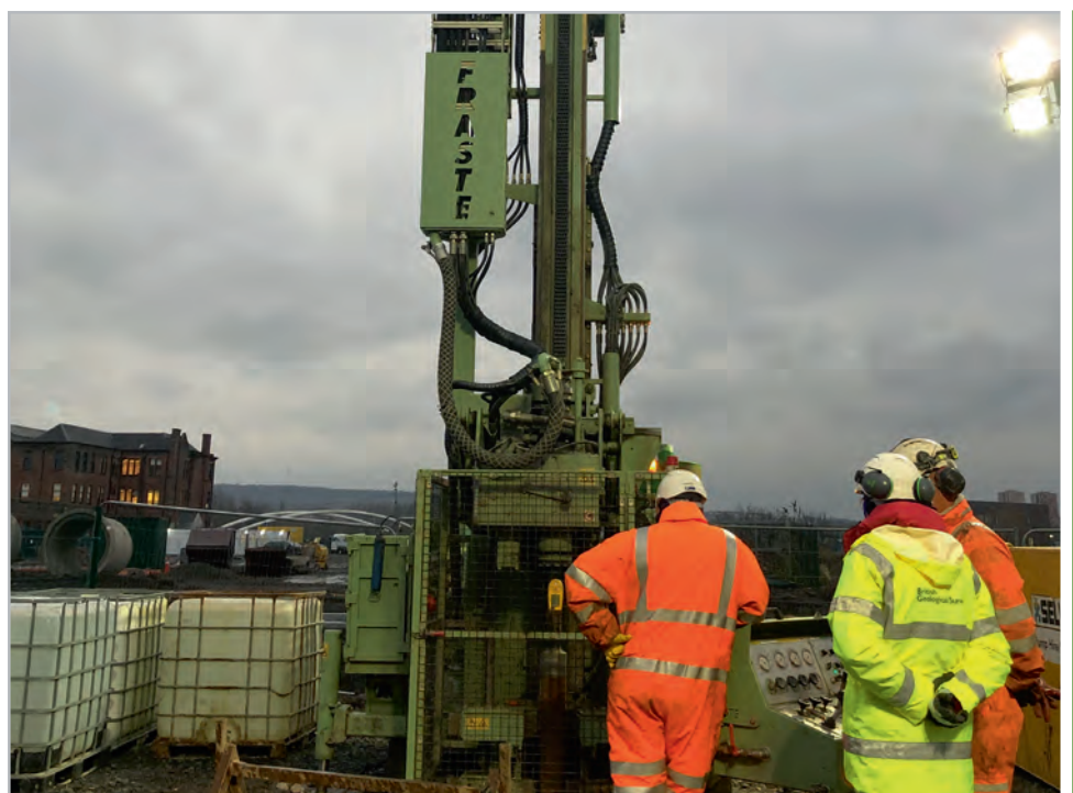
Drilling of the Glasgow Geoenery Observatory seismic monitoring borehole at Dalmarnock in November 2018. Photo number P987021 BGS©UKRI
