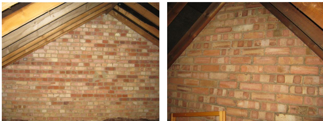
Figure 3.1: The brick pattern in the loft often provides clues about construction. Here, photo on the left shows a solid wall construction two bricks thick (notice the short 'header' bricks alternating in each course with longer 'stretchers'). The photo on the right is a full-height cavity-party wall (with all 'stretcher' bricks laid with the long side visible).
