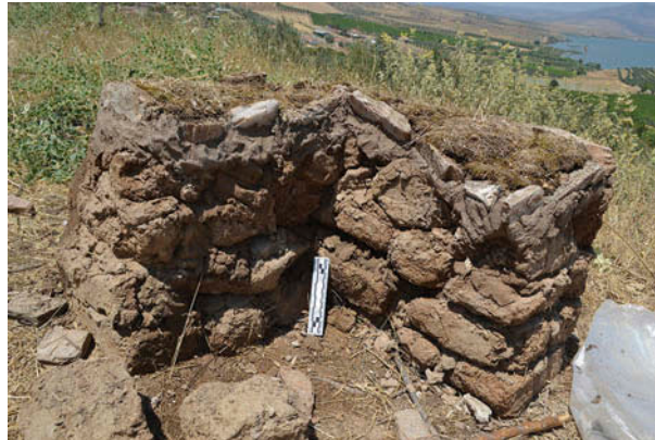
Figure 8. Soft vegetative cap applied Tekelioğlu experimental L-shaped mudbrick wall (top surface) directly after application.
