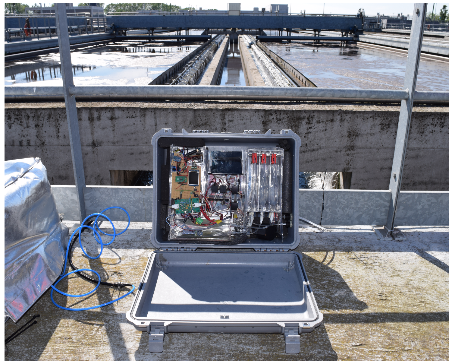
Nutrient Platform deployed after 2nd Stage Clarification at Milano San Rocco Waste Water Treatment Plant
