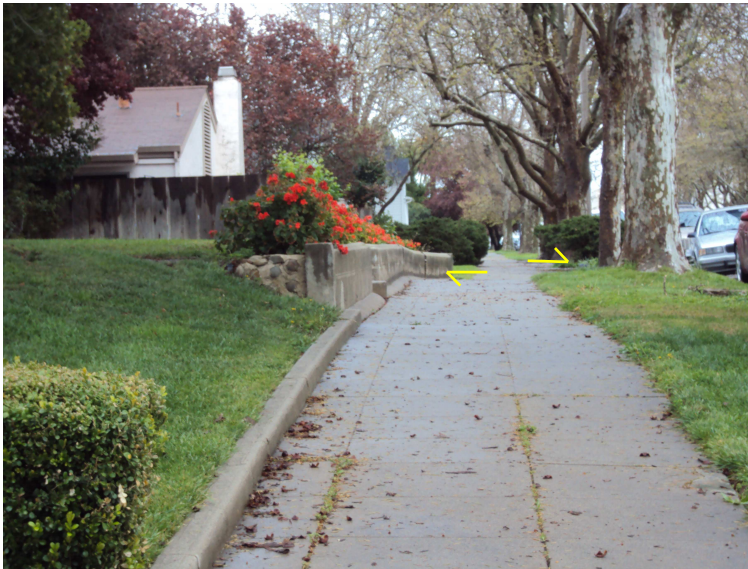
Figure 1.2: Image taken in Hollister, northern California, the slight bend in the pavement in the middle of the picture indicates the influence of the right lateral motion of the Calaveras fault (yellow arrows) which runs underneath the houses to the left. A large event is considered unlikely to occur in this particular section as it is creeping.
