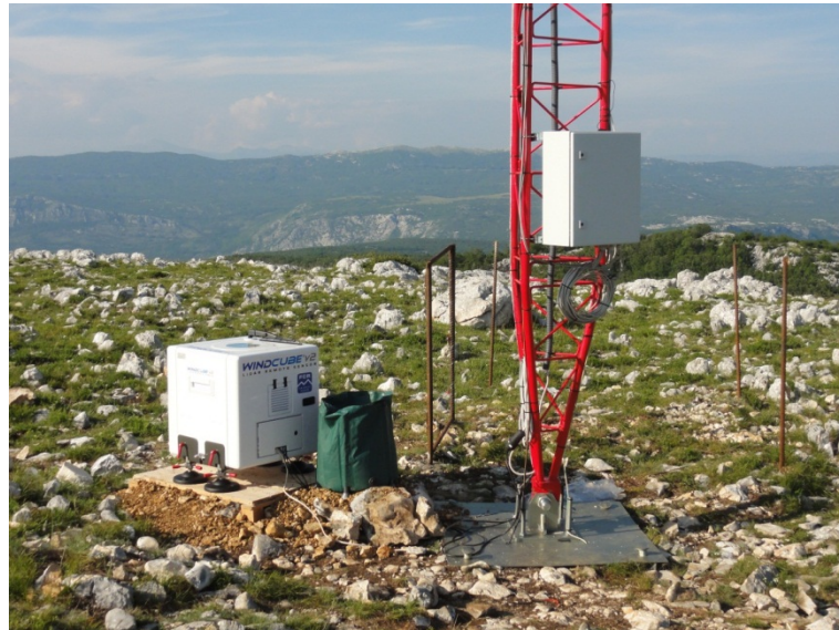
Figure 2 Picture of the lidar at 1.5m on the north side of the foot of the mast.
