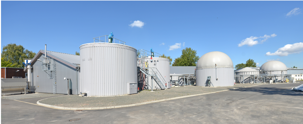
Figure 6: Overview of the DBFZ-Research Biogas plant ©Paul Trainer/DBFZ
